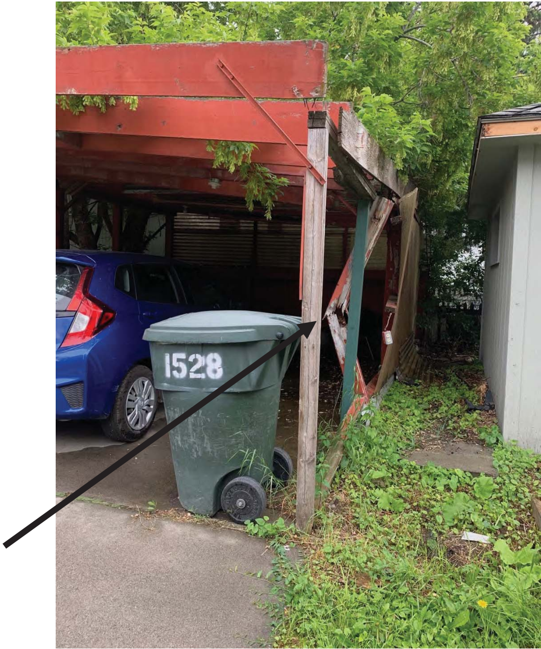
Exhibit XII. Photo showing additional information for the Board to consider. The current carport is deteriorating (supports are rotting/collapsing) and it needs to be replaced.
