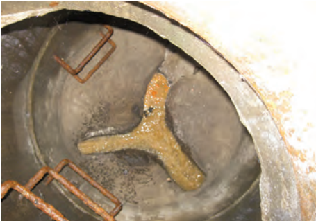
Grease clog in sewer.
