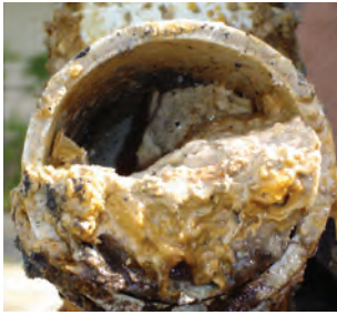
Grease clog inside a pipe.
