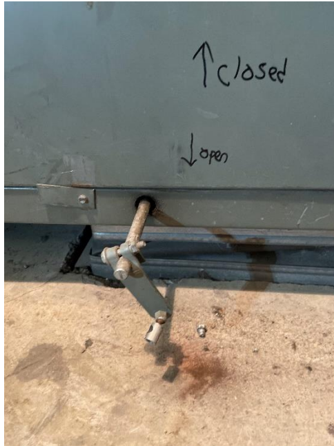
Figure 2 - Broken Damper Linkage
