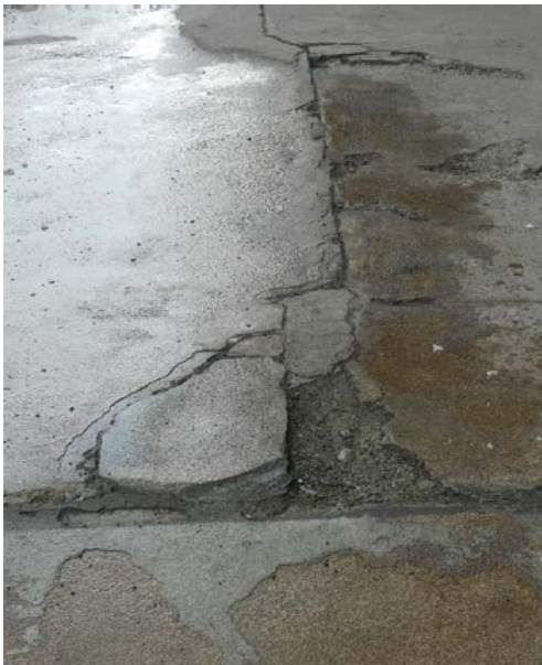
Sidewalk deterioration in study area
