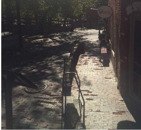
Missing Brickwork (Reeder's Alley)
