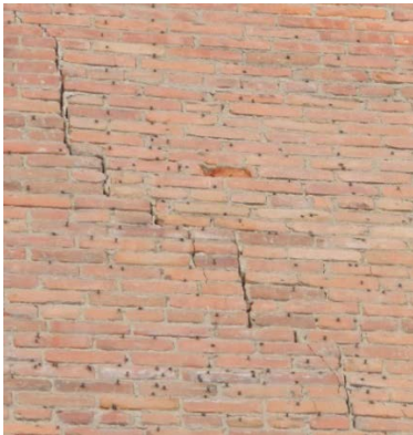
Bi-lateral cracking in building historic downtown core
