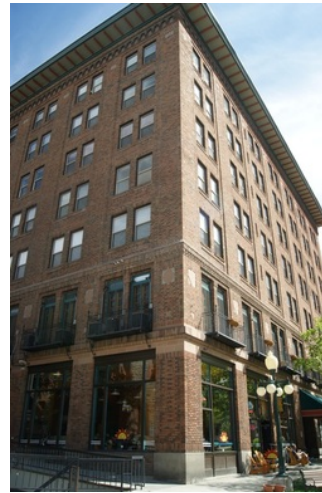
Example of a cornice at the top of the building (Placer Hotel)
