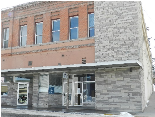
Building on Fuller Street with cladding removed on upper floors
