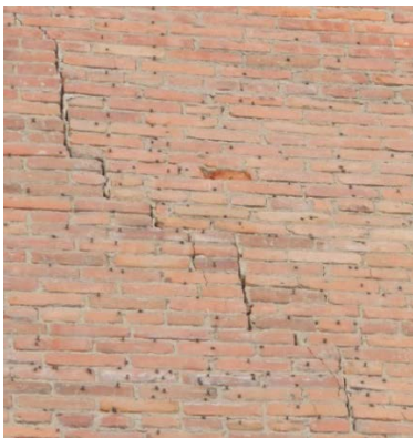
Bi-lateral cracking in building historic downtown core
