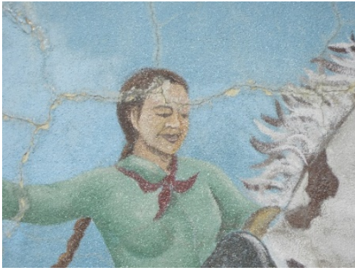
Cracking on Women's Mural
