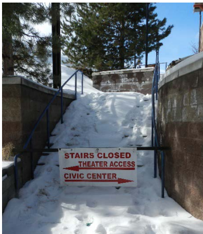
Unsafe stairway at Getchell Garage
