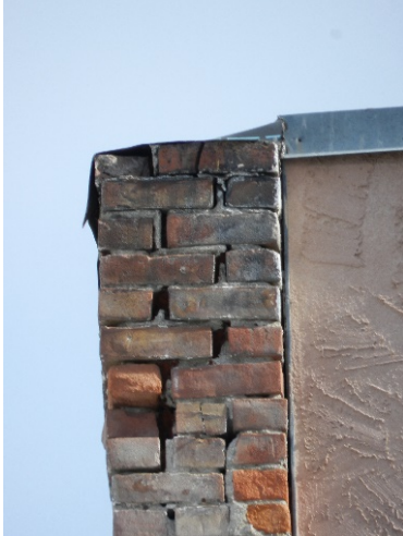
Brickwork that has lost mortar near the roofline of a downtown building
