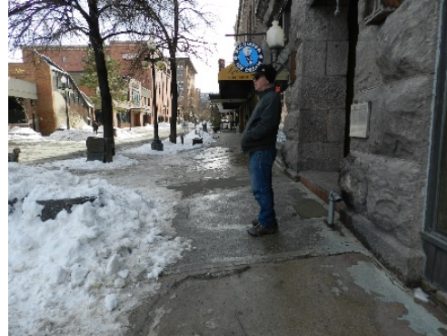
Sloped and cracking pavement in Walking mall
