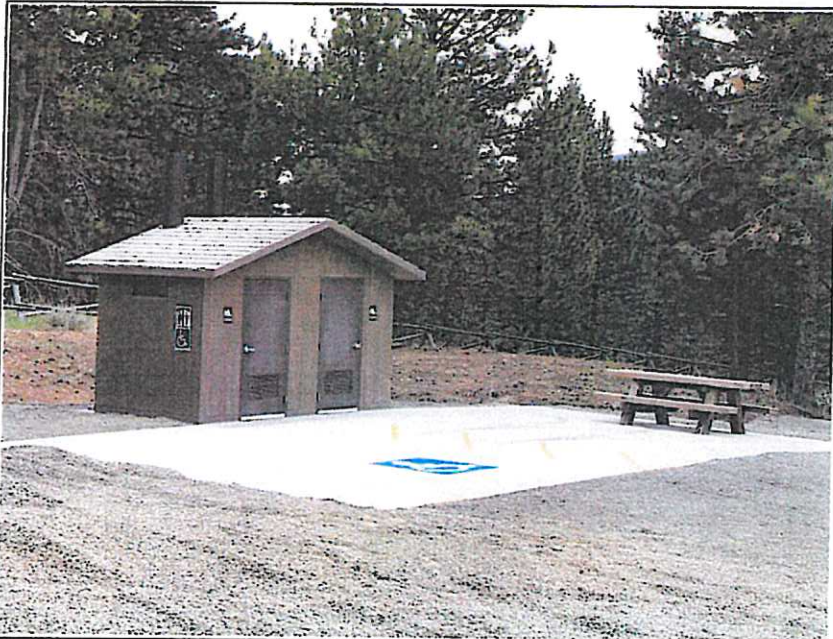
Park City Accessible Parking Pad installed at Park City Trailhead as part of a City of Helena/Helena Lewis & Clark National Forest Cooperative Project
