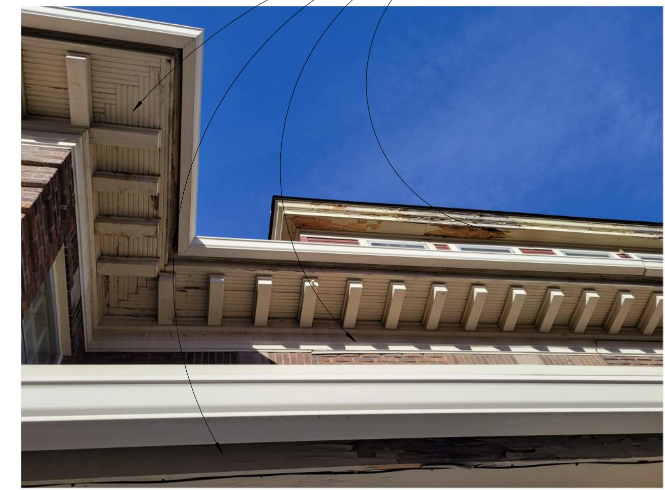
PORTION OF SOUTH ELEVATION - AT ROOF. TYPICAL DENTIL AND WOOD DETAILING AT ROOF SOFFIT
