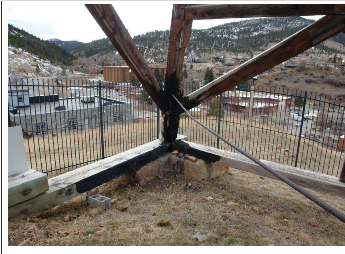
SW leg and bracing charred by arson in 2017
