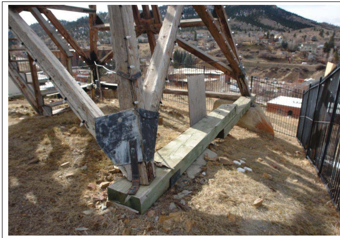
NW and NE legs with historically incorrect bracing, looking west
